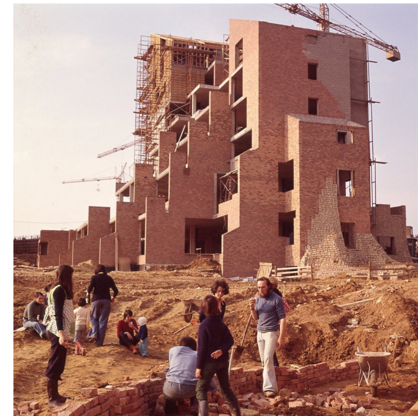
FIGURE 7: students working on the gardens during the construction work (photo: Louis le Roy)
